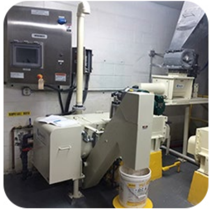
Nebraska City WWTP, NE
