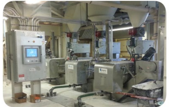
Davis WTP, Austin TX
